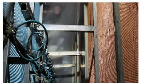
KT&G Air Conditioner Humidification Control System
